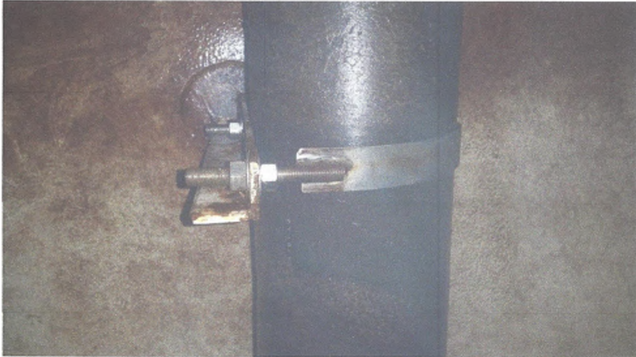
(8) Second bracket on the Intake Pipe.
