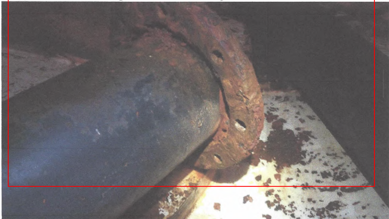
(7) Corrosion on the Flange on one of the intake Pipes.
