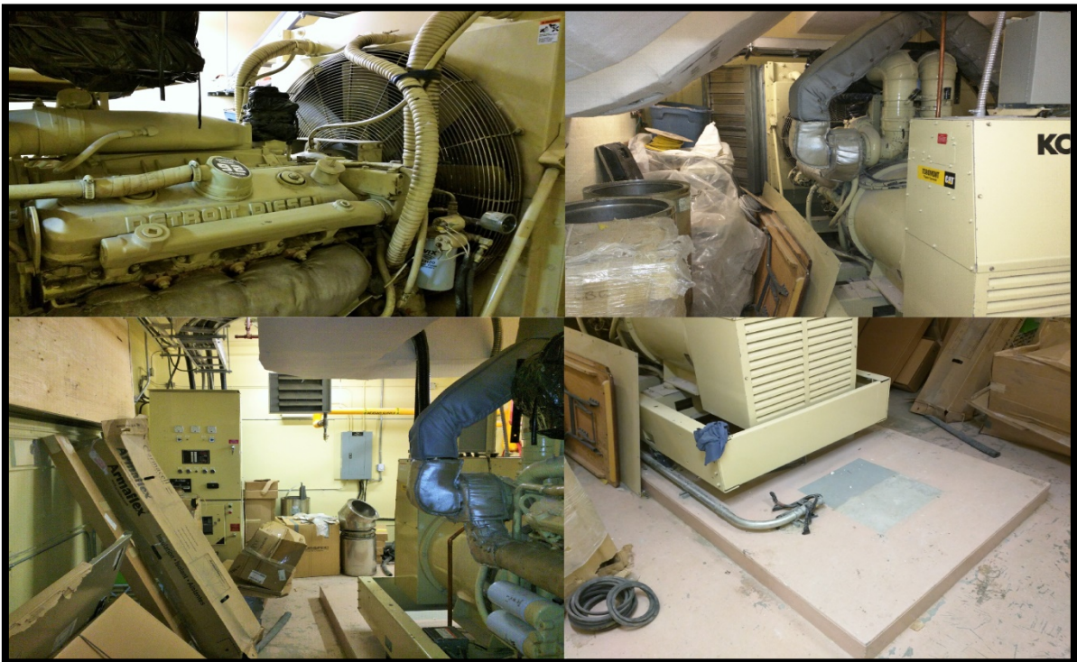
Figure 3: Generator, generator controls and riser.
